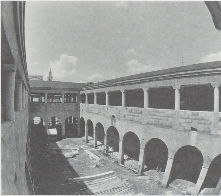
Fish-eye view of the Cornell Hall courtyard under construction during the summer.
